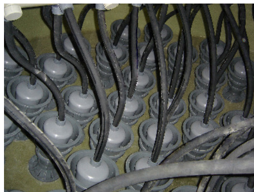
Multiple Ring-Jet modules installed in parallel in a scrubber
